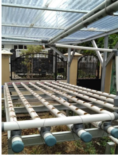
Figure 8. Hydroponic Plant Pipe
