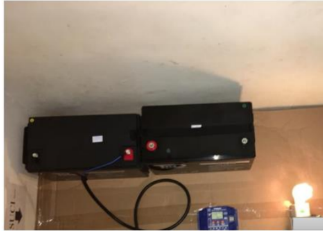
Figure 6. Battery Installation (Dry Battery) with Solar Charger Controller
