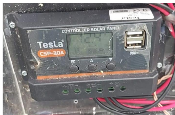
Gambar 4.12 Pengujian Solar Carger Controller
